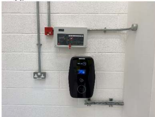
Car Charging point
